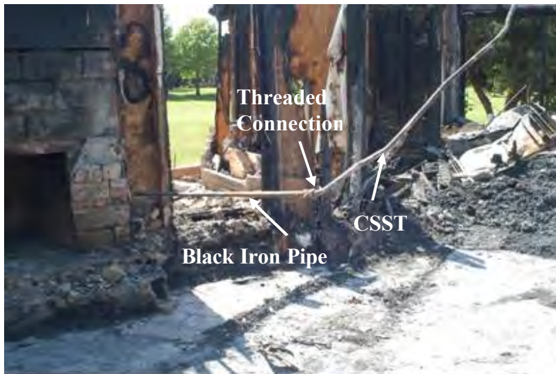
Figure 5: CSST tied to Black Iron pipe from fireplace
