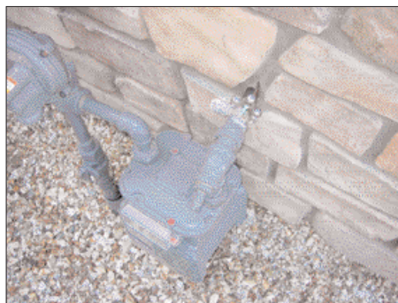
Figure 1: Bonding Clamp at Gas Meter Outlet
